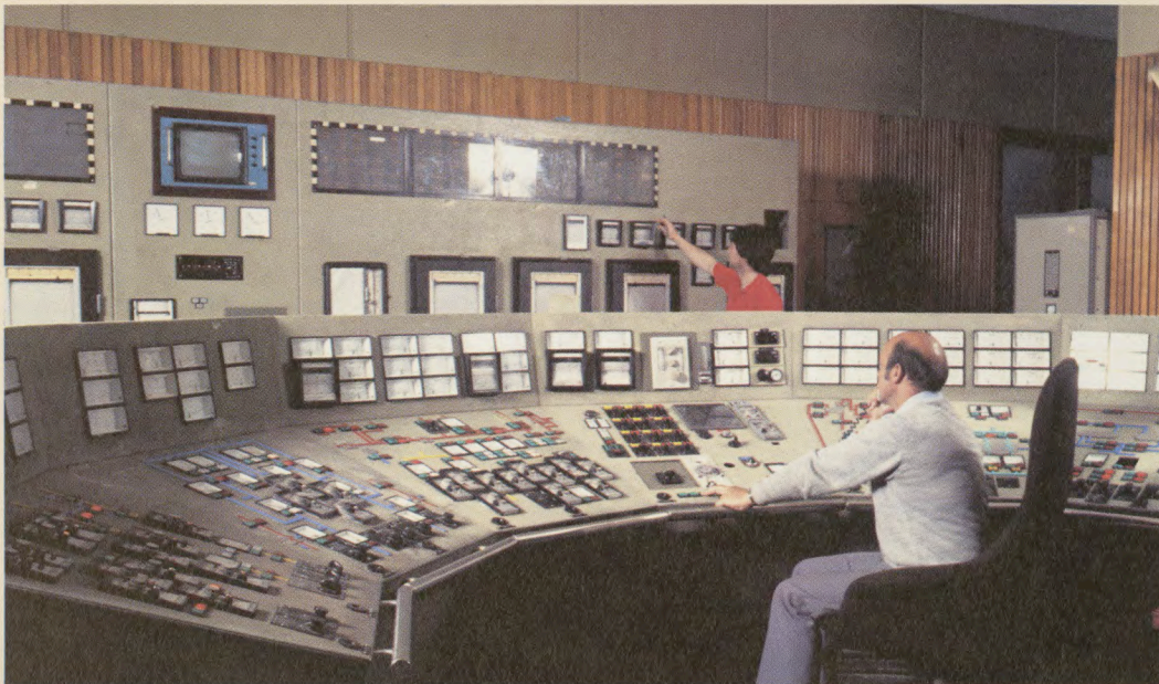
Electrical Control Room.
