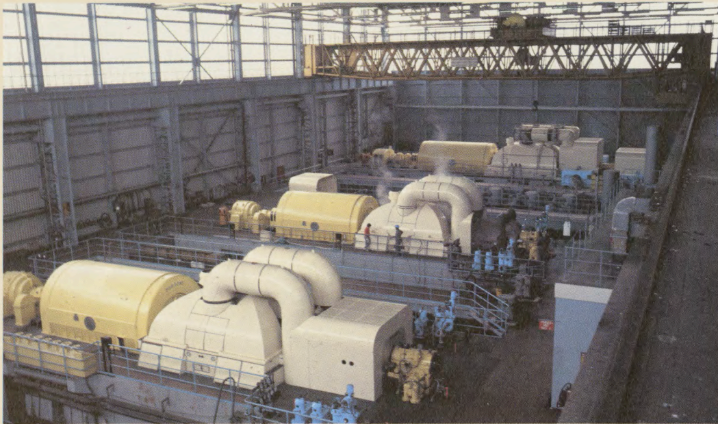
The Generating Hall.
