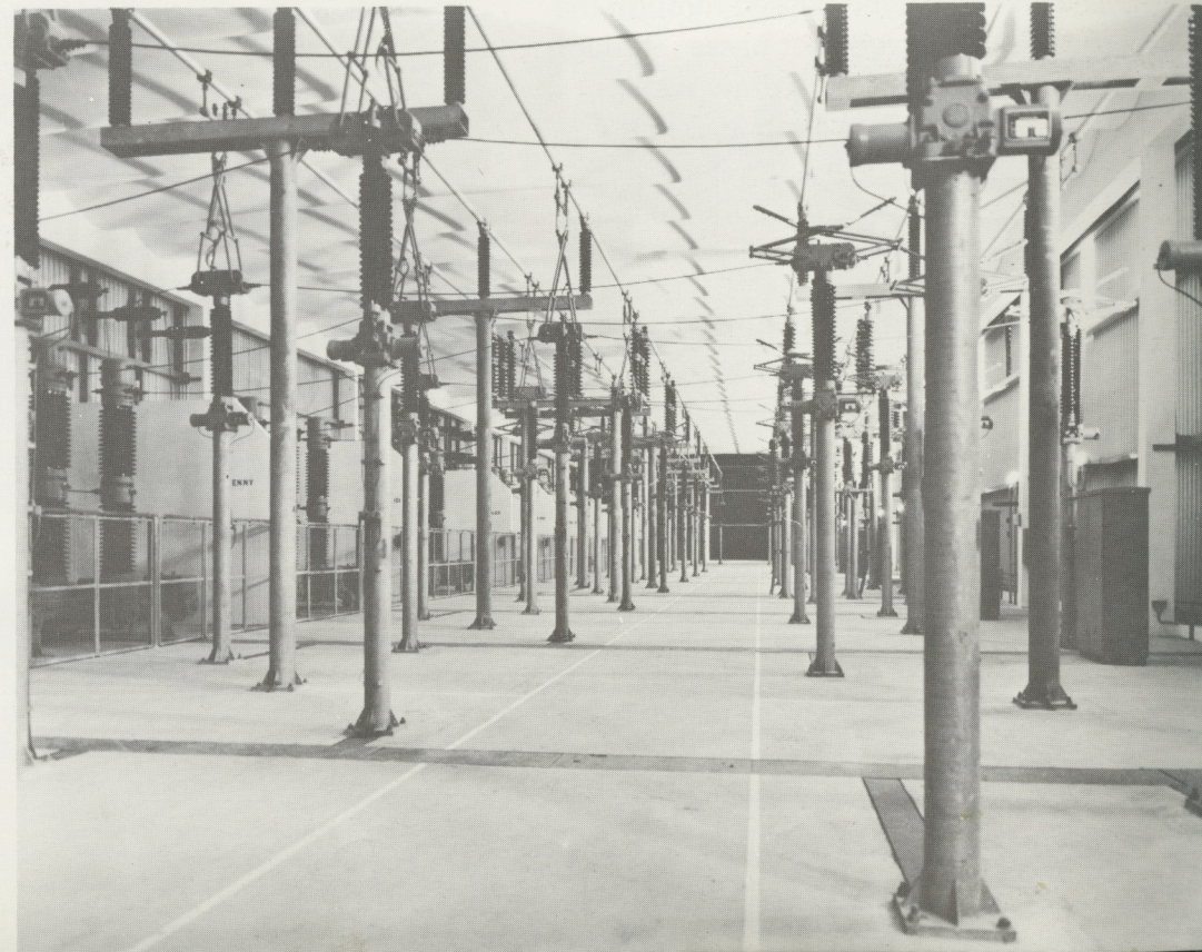
The Indoor 110 kV. Transformer Station.
