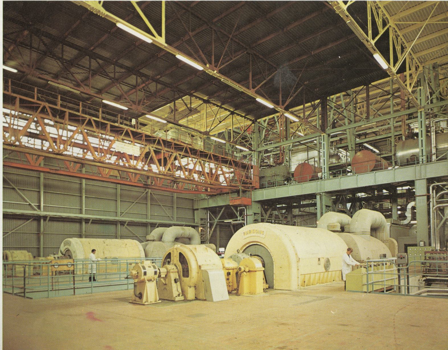
The Thermal Control Room (left) and the Generator Hall (right).
