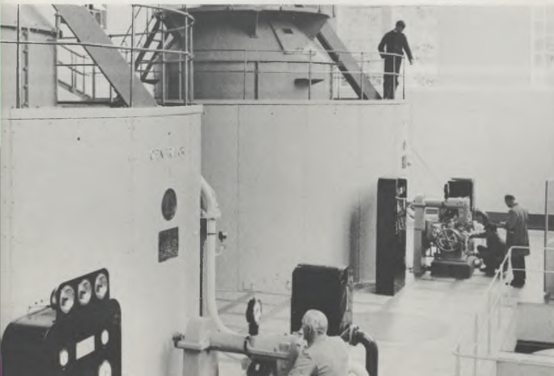
Below: Generating Hall
