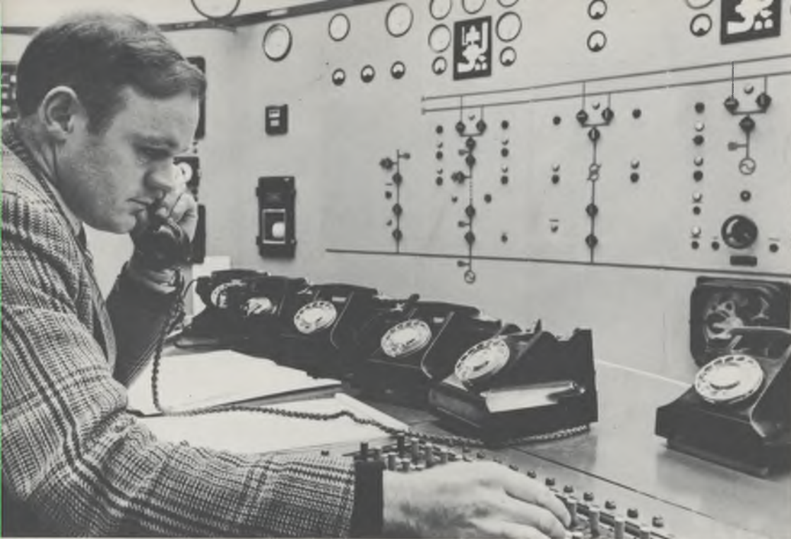
Above: Control Room
