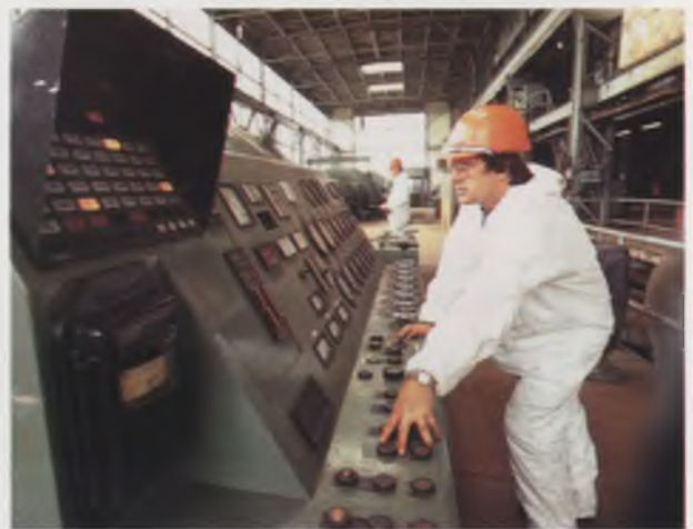
Turbine Control Panel
