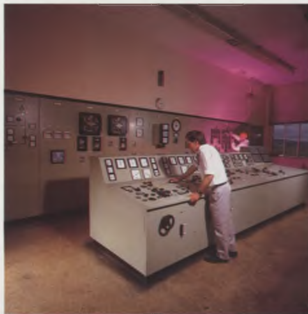
Electrical Control Room
