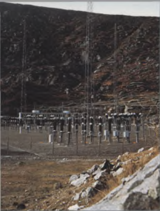
The 220KV switchyard.
