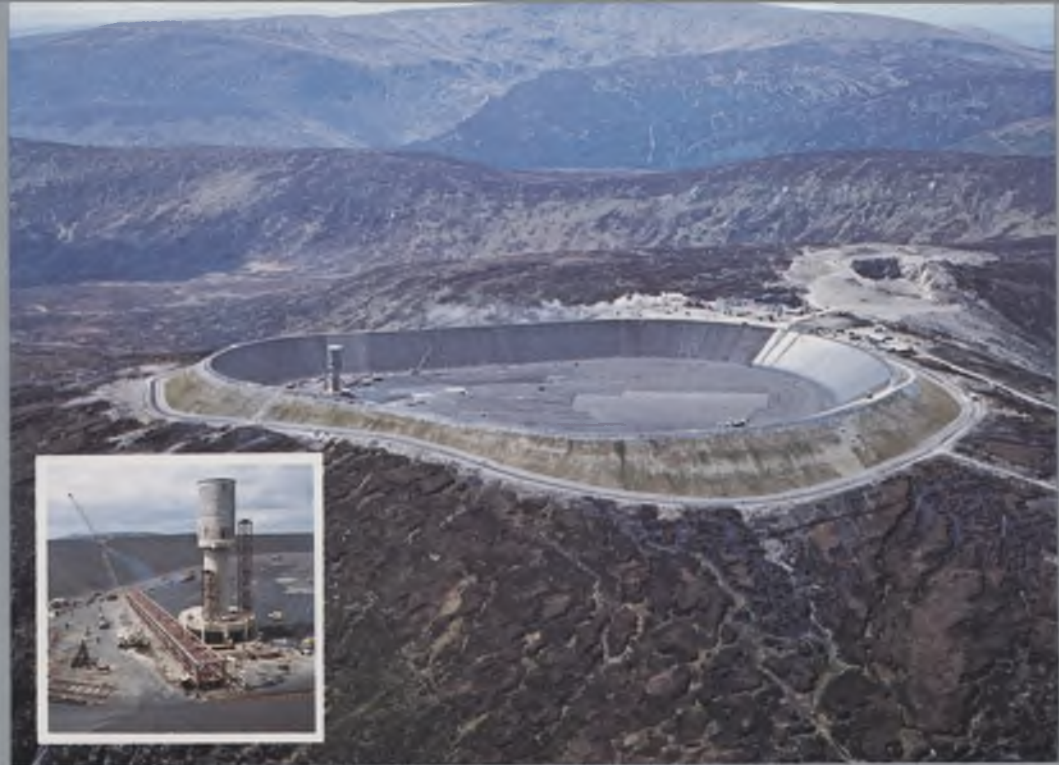
The upper reservoir under construction with an inset showing the intake structure.
