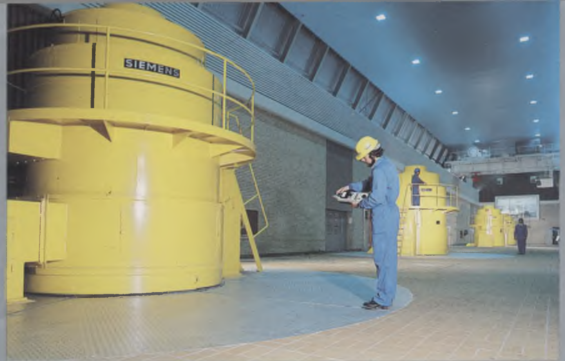
The generating hall showing the four 73MW pump-turbines.
